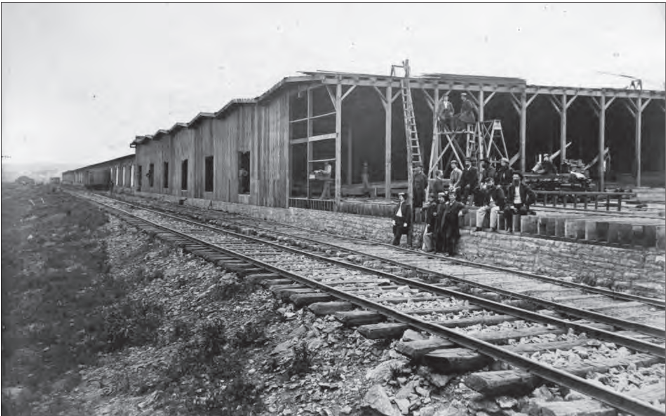
Unfinished forage house on N&NWRR in Nashville with a group of officers of the Quartermaster Department. The facility was to be built in two sections — 904x156 and 805x112. Only 201 feet of the second section had been completed. A forage house was used to store hay and oats for the Army's horses and mules. (Tennessee State Library and Archives.)
